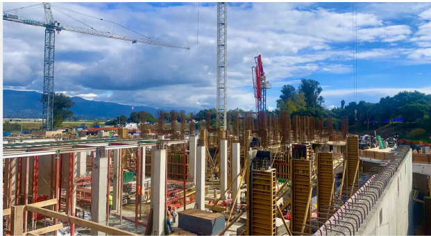
Photo Credit: Kristen Brinlee Work on the San Benito Student Housing Project began in spring 2025 and is on schedule for anticipated occupancy in the fall of 2027.
